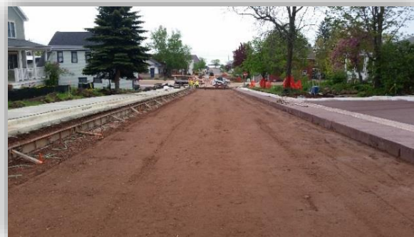
Modern subbase and drainage facilities were installed to filter sediment and reduce the pollutant burden on nearby Lake Superior.
