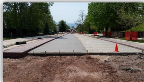
A concrete base layer with weeper holes was constructed to support and prevent potential frost damage to the vintage brick surface.
